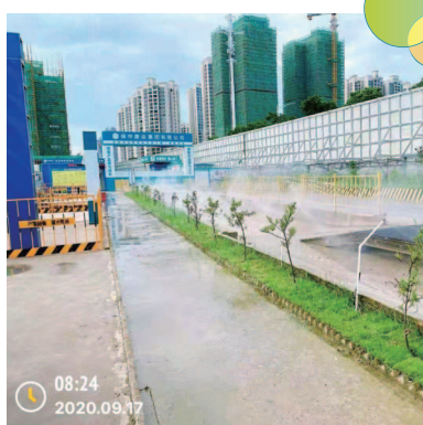
Roadside Dedusting Spray
